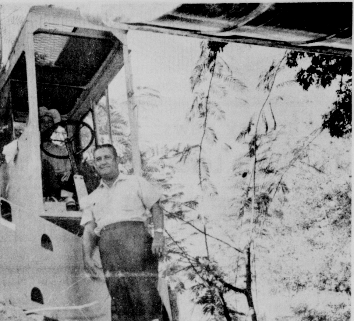
WORM'S EYE VIEW - Gregg County Commissioner Bill Owens guides the movement of the big Drott backhoe into the ditch on Jeannette Street where the county is assisting the city in putting in storm drains. The Canfield-Jeannette Street area has long been plagued by flooding during heavy rains. The new drains will relieve the situation. The backhoe is operated by county employee Bill Bailey of Greggton. The scoop was about to take a bite when this photo was snapped.
