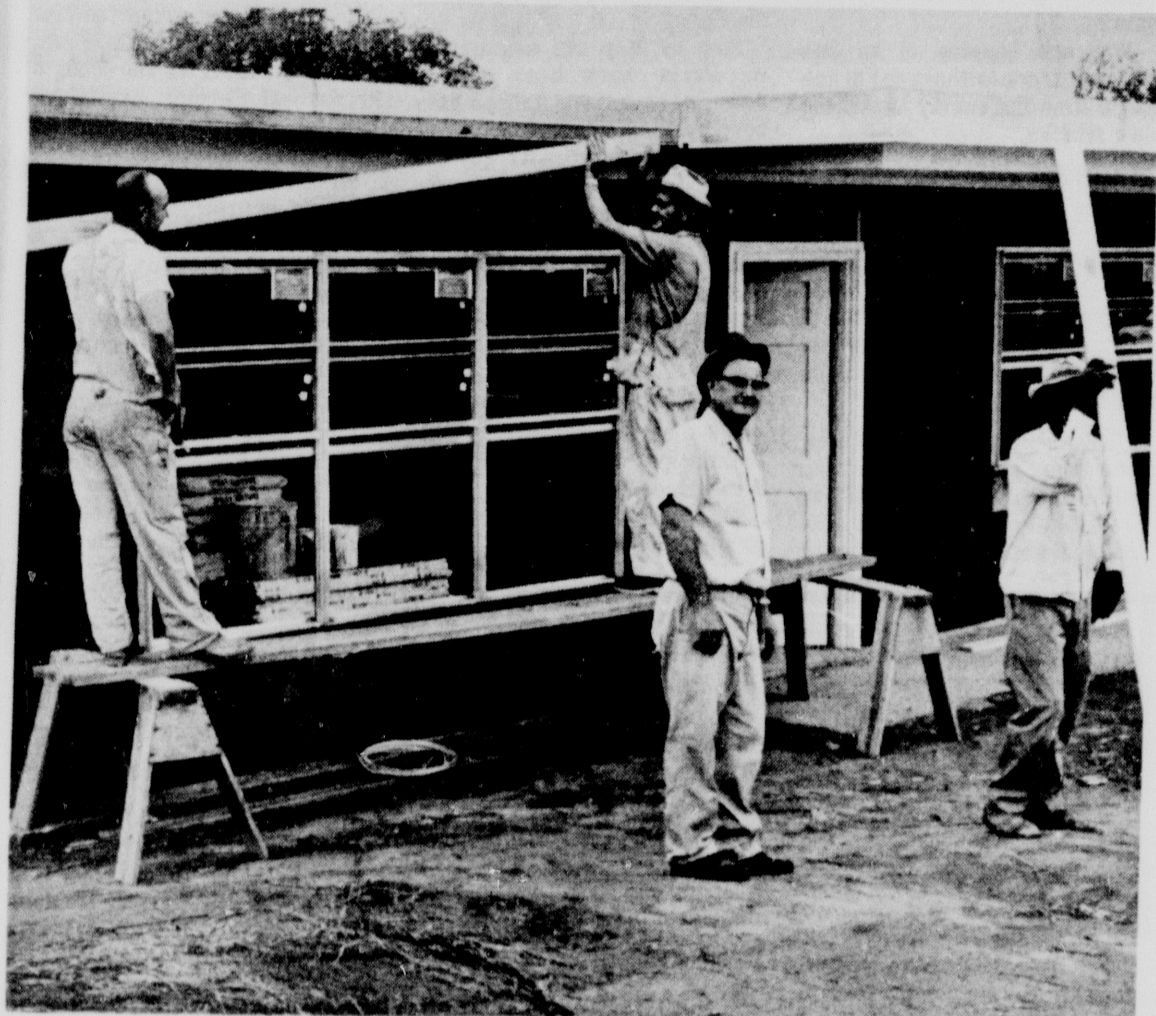
FIRST BUILDING - Gladewater builder A. B. McPherson, center, and son Bobby (at left with plank) work on the first unit of a planned four-building apartment development. Each building will have four two-bedroom apartments, a total of 16. McPherson said this first unit should be completed by September 1. The development is adjacent to the Oak Manor Nursing Home on East Broadway (Highway 80).
