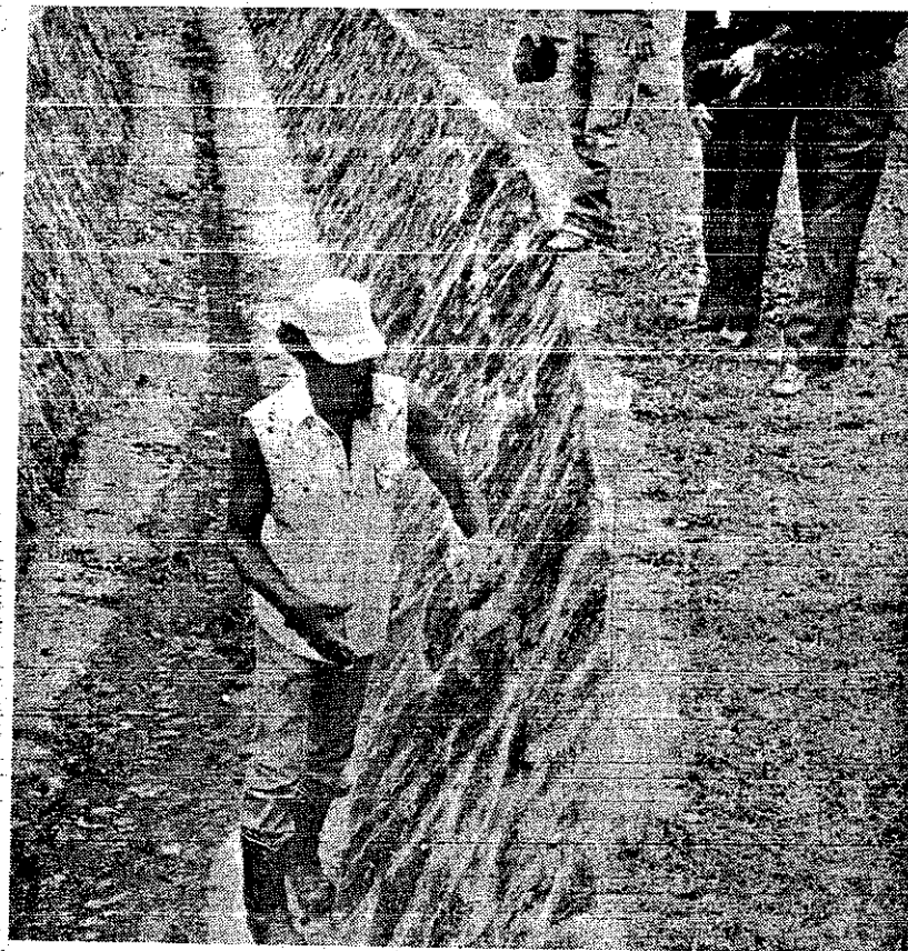
ROCK WORK — An employee from Saylor's Masonry in Longview puts the finishing touches on some rock work in the City Park as the owner of the company, Nelda Lewis and Virginia Long look on. The firm, at the expense of KIBA, replaced and repaired the rock in the creek running through the park. KIBA adopted this project several years ago and has now seen it completed. Mrs. Lewis and Mrs. Long are active in KIBA, with Mrs. Long serving this year as president. The group also has the park as its Adopt-A-Spot. (Photo by Greg A. Collins)
