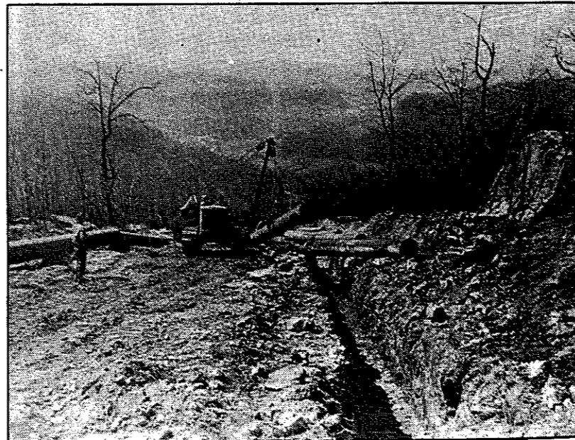
This historic photograph from Dr. Norman Black's collection was taken during construction of the Big Inch pipeline during World War II. Recognizing a need for an overland oil route — the United States was losing almost three tankers a day in 1942 — the pipeline was built between Longview and Norris County Ill. to carry oil to the east coast.
